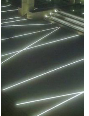
In ground lighting
