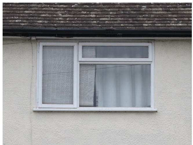
Inappropriate Window design
