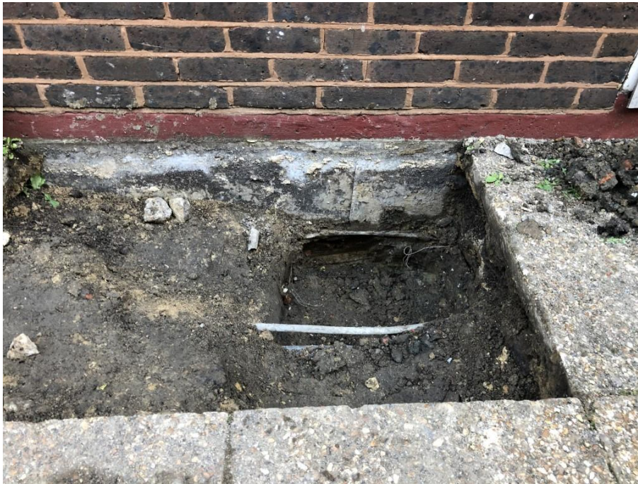
Ground slab bearing on made-up ground at 83 Manor Grove
