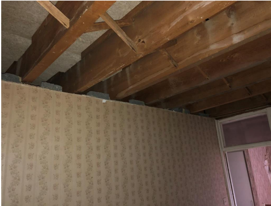
Photograph 7 – Roof structure spans between load bearing flank and party walls at No. 81. Non-load bearing blockwork partition visible.
