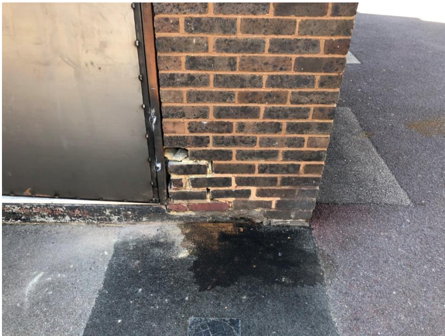
Photograph 4 – Low level brickwork cracking at No. 81.
