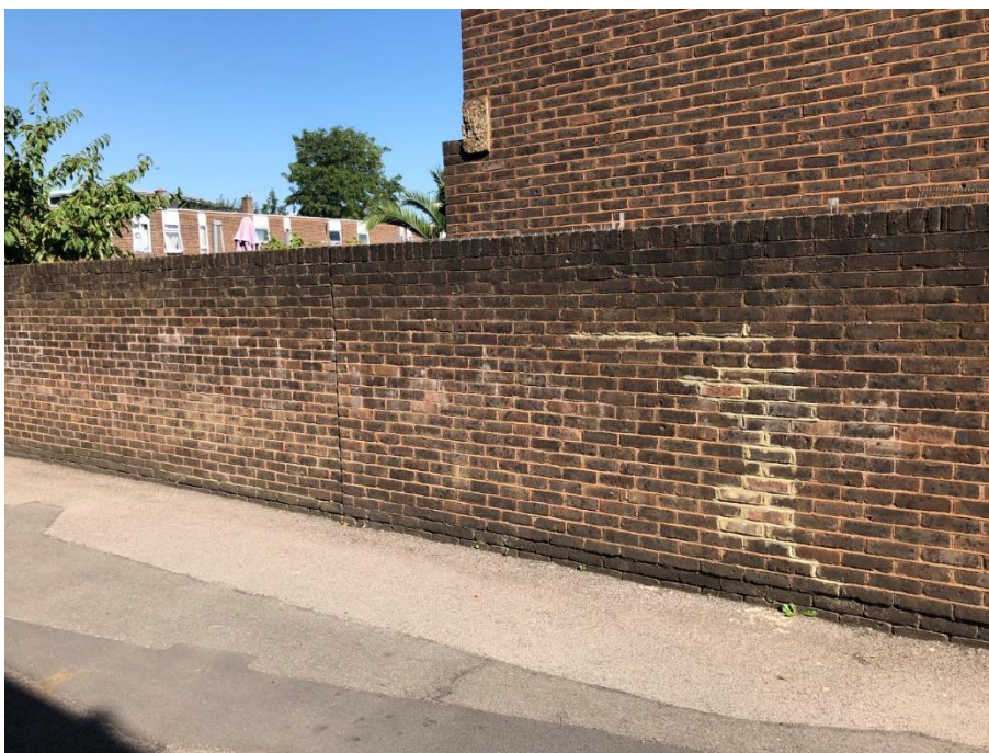
Photograph 16 – Boundary wall with movement joint. Note repair and lateral displacement at damp proof course.
