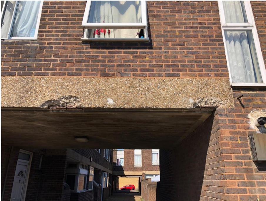
Photograph 11 – Spalling reinforced concrete slab edge.
