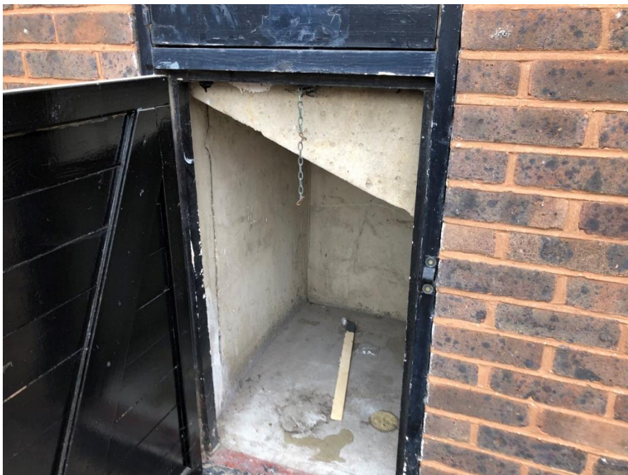
Photograph 6 – Concrete lining to under-stair cupboard. Vertical crack indicates junction with brickwork.
