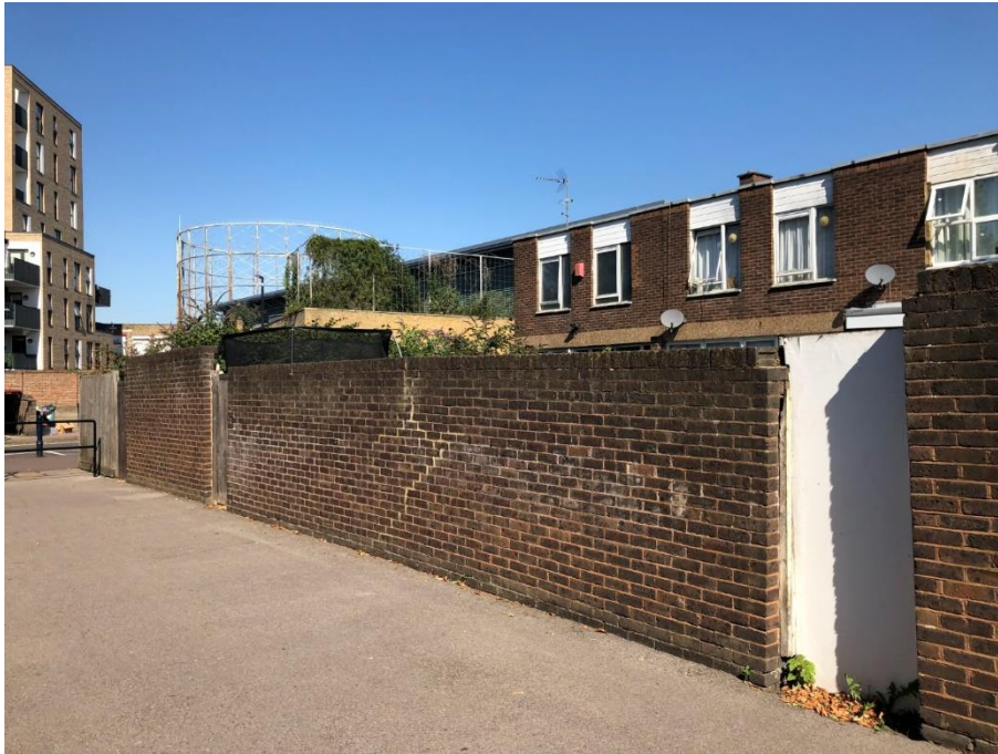
Photograph 15 – Typical cracking to boundary walls.
