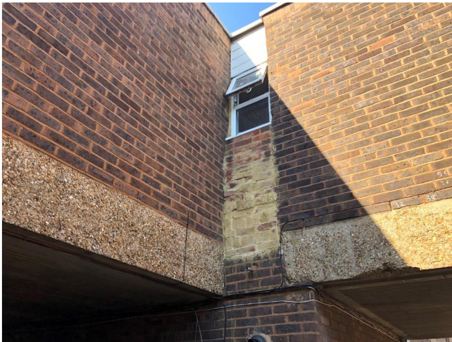
Photograph 14 – Poor quality infill brickwork to window openings. Comparable window openings elsewhere appear to be full height, as this was assumed to have been.
