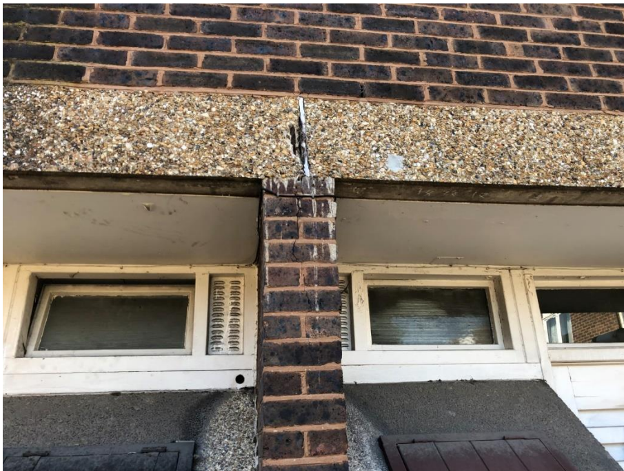
Photograph 12 – Vertical cracking through brickwork at supports to concrete elements.
