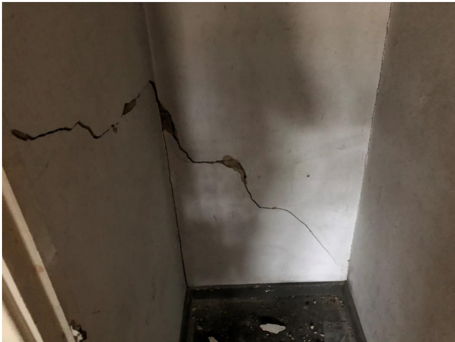
Photograph 10 – Internal cracking at understair cupboard reflects that viewed externally.
