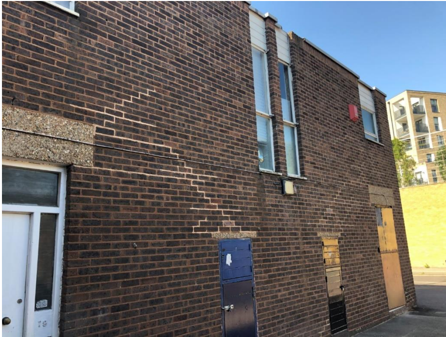
Photograph 3 – Typical pattern of cracking at Nos. 79 (near) and 81 (far).
