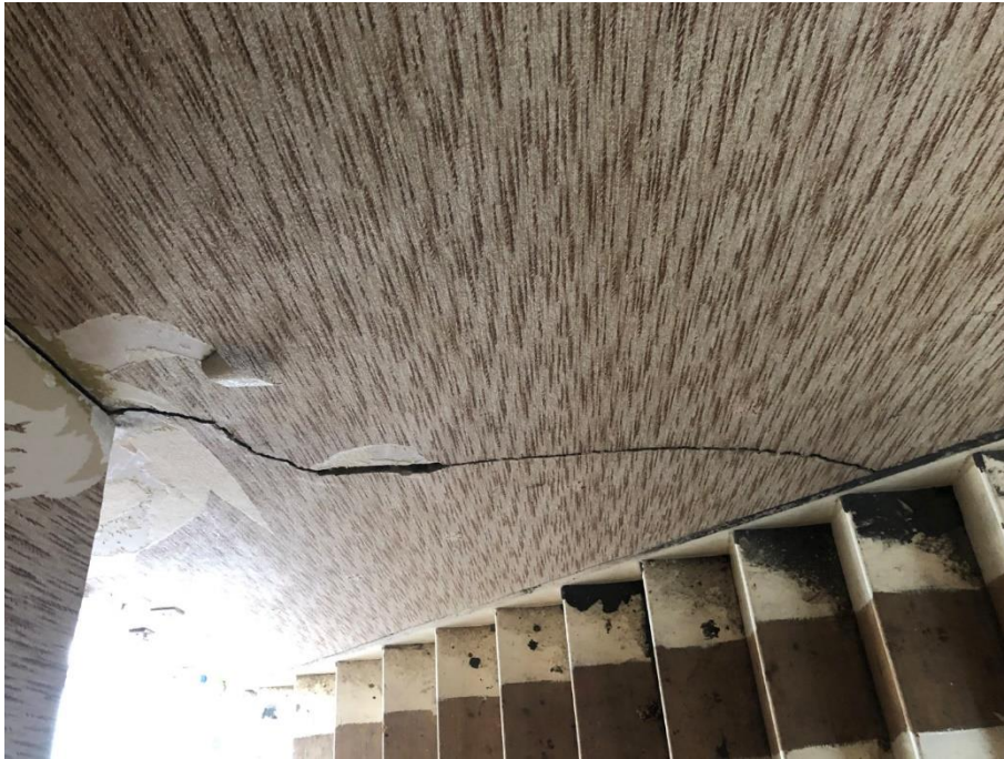
Photograph 9 – Horizontal crack across stair reflects horizontal cracks in external brickwork.
