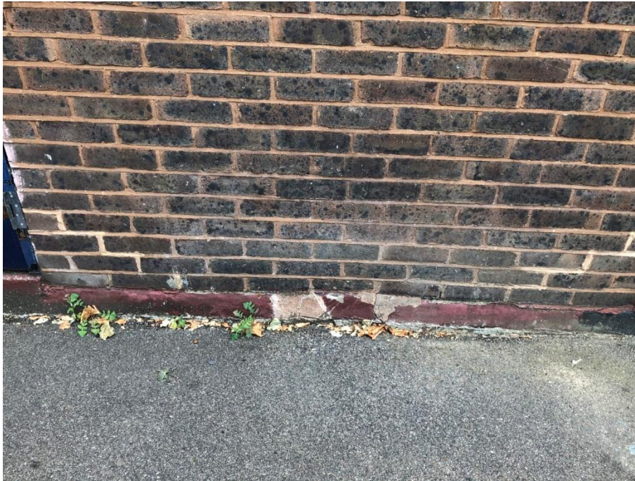
Photograph 5 – Cracking at ground level indicates junction between load bearing party wall and ground floor slabs. Note diagonal cracking to brickwork on both sides.
