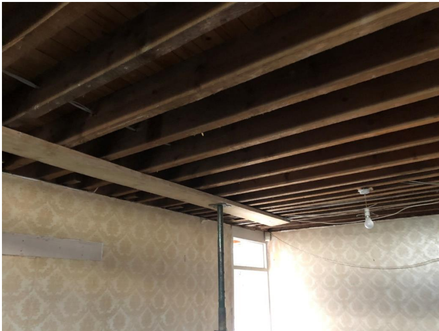
Photograph 8 – First floor joists span from load bearing walls to central supporting wall. Note spacing of joists reflects intensity of loading.
