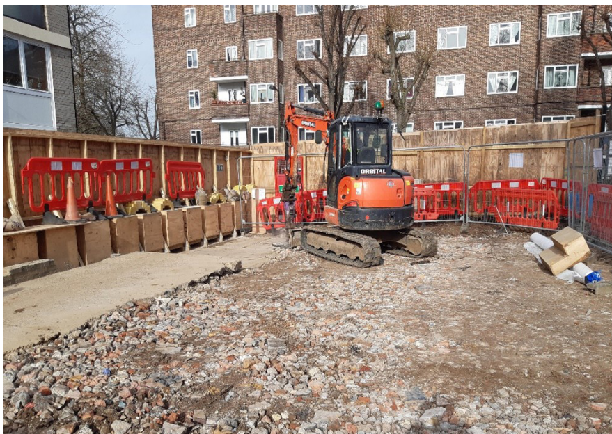
Breaking out of concrete slab and lower section of site piling mat
