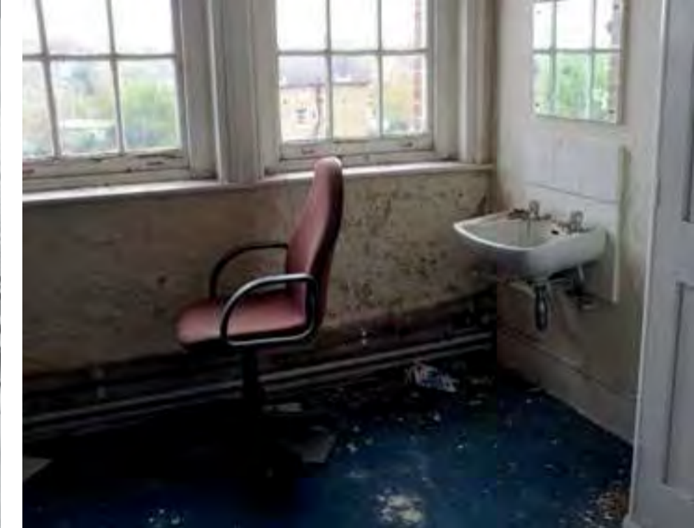
The 2 of 4 remaining ward buildings are in a poor state of repair
