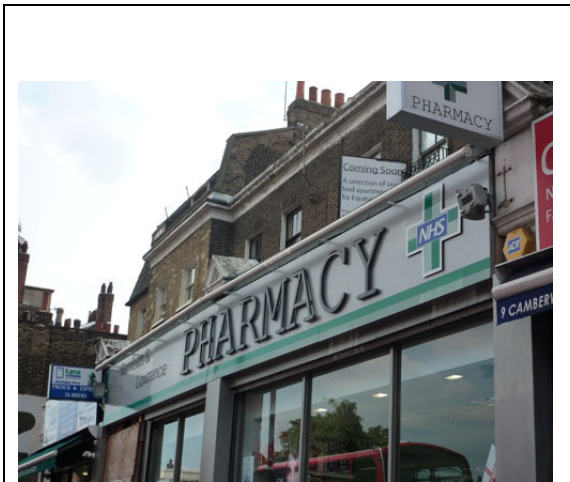
Camberwell Road: Inappropriate modern fascias can detract from the overall quality of a building
