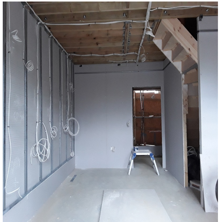
Block A The Townhouses – Block A showing The staircases installed and internal walls are 1 st fixed and plaster boarded one side. Also Mechanical and Electrical 1 st Fic is complete
