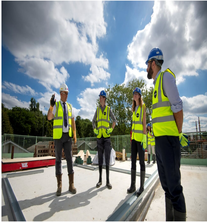
Block B The Apartments – Standing on the 2 nd floor as the Metal walls were commencing to form the apartments on Level 2.
