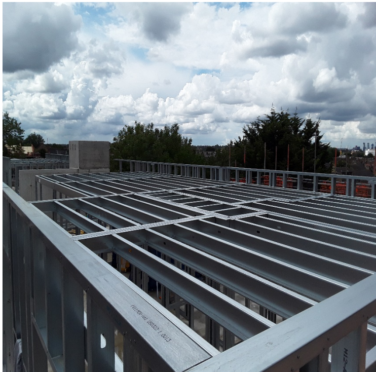
Block B The Apartments – Standing on the 2 nd floor now the Metal walls are almost complete forming the apartments on Level 2.
