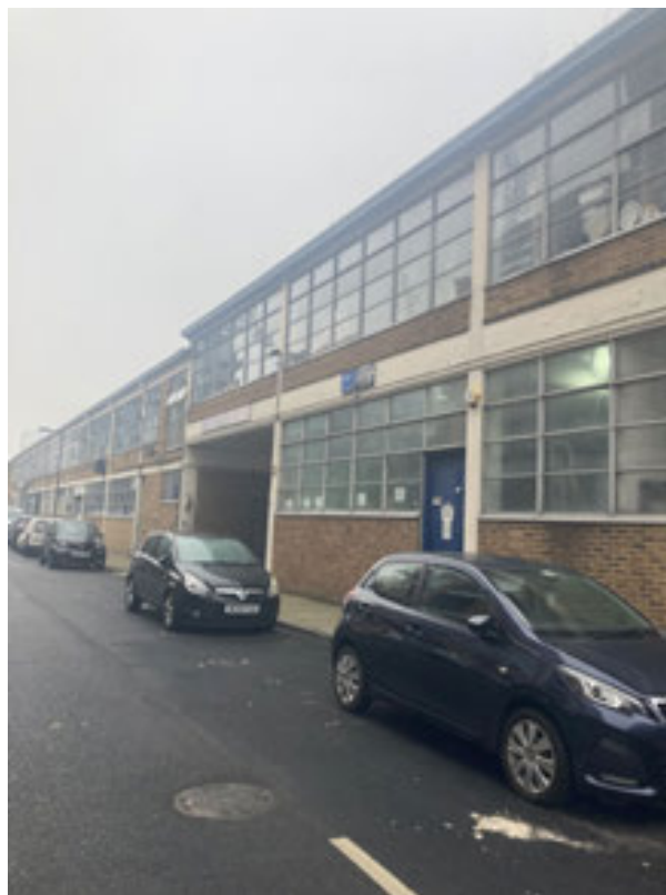
Plate 16: The Penarth Centre on the west side of Hatcham Road, a two storey light industrial facility probably constructed in the late 1950s with brick and block elevations around a reinforced concrete frame. Note the original windows and door elements.
